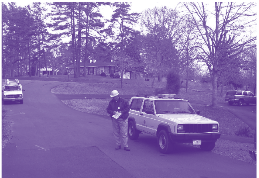
Bernie Wilson, Anderson County Encroachment Inspector, ensures that proper procedures are followed during a road cut repair.
