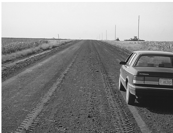
It is very important to establish correct shape on surface prior to placing new gravel. The reshaped surface should have same crown as finished gravel surface so that a uniform gravel thickness will exist on the road.
