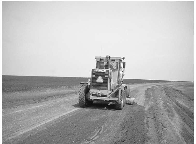
Motorgrader doing final shaping on fresh surface gravel. The road now becomes much easier to maintain in the future.
