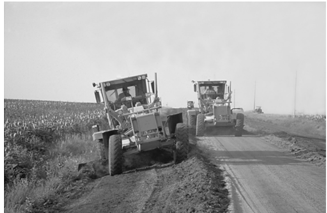
Good example of reshaping techniques. Motor-grader should be used either on inslope or on surface to maintain a shoulder line.
